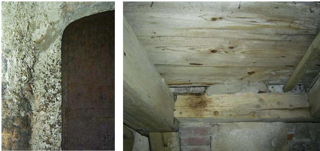
Fig. 4-21: Gaps through which the animals can slip into and out of the roost: between a door and a wall (left) and at the base of the roof (from the outside the animals appear under the eaves gutter). The place where the mouse-eared bats land on the wall and beam is discoloured brown. Photos: A. Zahn
