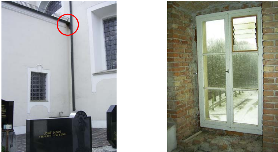
Fig. 4-22: Ingress passage below the guttering, identifiable by the dark discoloration of the wall (left), and ingress passage through diagonal window slats (right). Photos: A. Zahn
