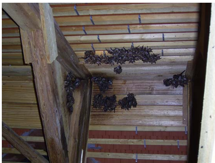
Fig. 4-24: Boards fitted at the ridge of Frichlkofen Church (Bavaria, D). The seamless rabbit and feather joints (tightly sealed at the ridge), enable warm air to build up. From as early as the first year, the animals hung from the new boards. Photo: A. Zahn
