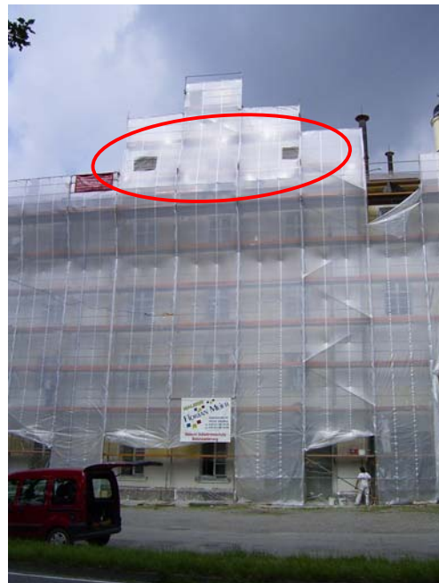
Fig. 4-17: The egress openings of the colony of Geoffroy's bats, consisting of about 250 animals, is located on the top floor of the attic. In 2005 the facade was renovated. Photo: A. Zahn
