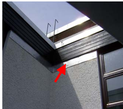
Fig. 4-30: Metal sheeting “bat repellents”, to prevent noctule bats flying in above house entrances (Wasserburg, Bavaria, D). Photo: A. Zahn
