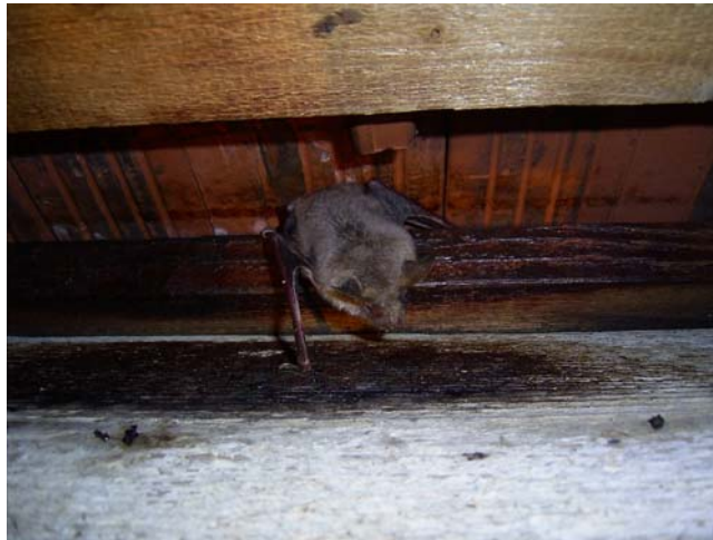
Fig. 4-20: Brown discoloration of wood, brick and wall at a hanging place of male mouse-eared bats. Photo: A. Zahn
