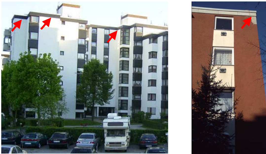
Fig. 4-28: Roosts of noctule bats behind wooden panelling (Wasserburg, Bavaria, D, left), and asbestos cement panelling (Waldkraiburg, Bavaria, D, right) at the edge of flat roofs. Photos: A. Zahn
