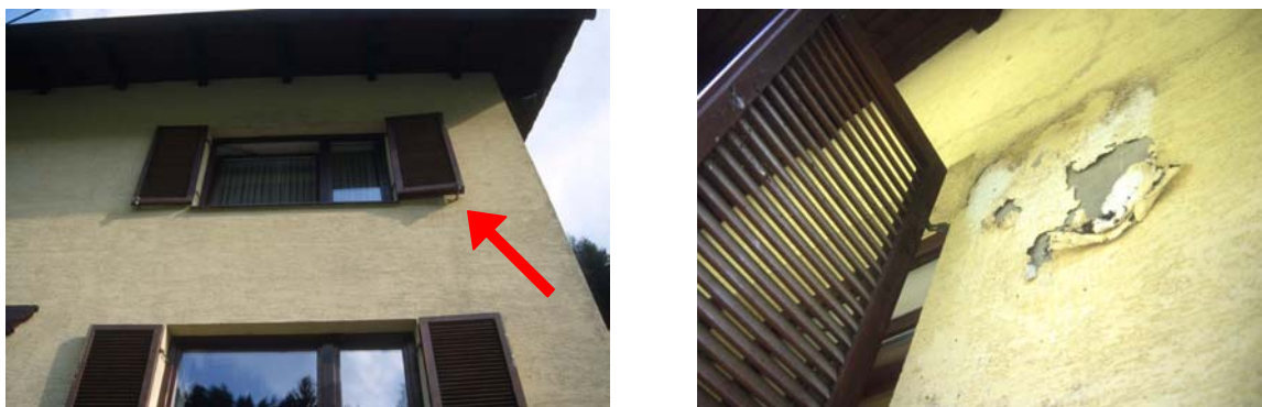
Fig. 4-42: Damage to a wall façade caused by the urine and droppings of a Barbastelle bat nursery behind a window shutter (Bad St. Leonhard, Carinthia, A). Photos: M. Jerabek
