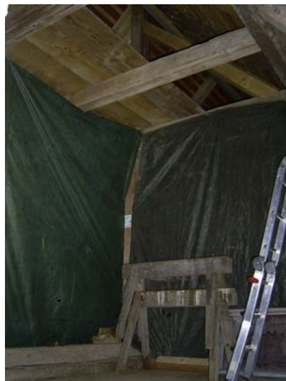
Fig. 4-23: Partitioning off the hanging places with dark sheeting, at Kläham (Bavaria, D). Photo: A. Zahn
